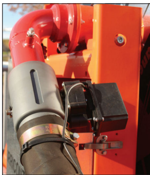
Butterfly valve controlled by electric motor
